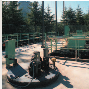
Water treatment facility
